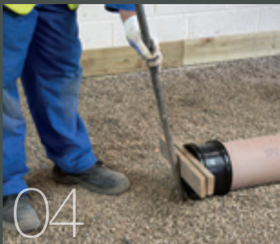
Larger pipe sizes can be jointed with the assistance of a bar
