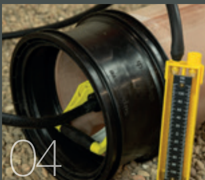
04 Apply pressure to achieve a 110mm water gauge on the manometer
