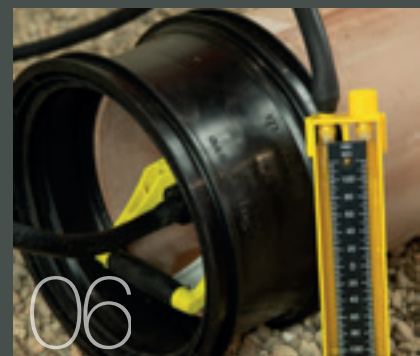
06 Measure the pressure drop over a period of 7 minutes
